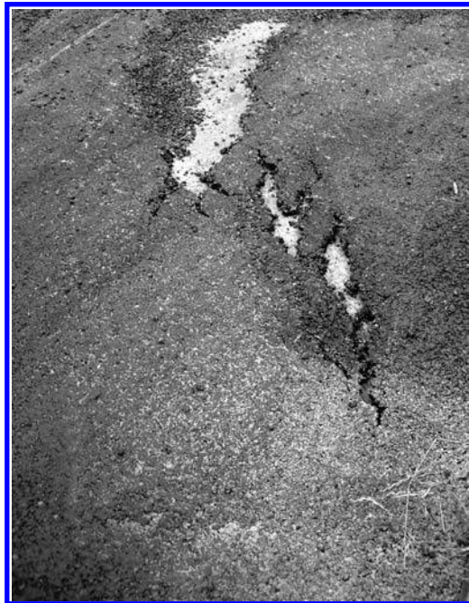
FIGURE 11.32 An example of the tearing of an SMA mat due to the lack of a tack coat on the cement concrete bottom layer. (Photo courtesy of Krzysztof Błażejowski.)
