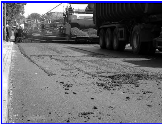
FIGURE 11.33 Remains of mixture left on a bottom layer resulting in unevenness of the finished course. (Photo courtesy of Krzysztof Błażejowski.)
