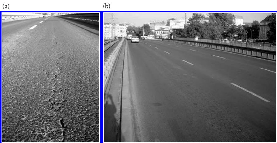
FIGURE 13.2 The bridges in Płock and Wrocław: (a) condition of the Płock bridge pavement; (b) condition of the Wrocław bridge pavement. (Photos courtesy of Krzysztof Błażejowski.)
