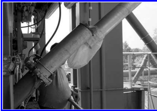
FIGURE 9.10 Performance inspection of the granulated stabilizer batching into a plant's pugmill. (Photo courtesy of Krzysztof Błażejowski.)
