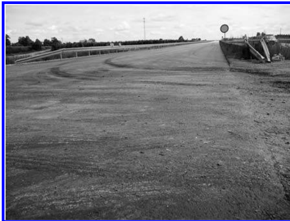
FIGURE 10.6 Soiling of an intermediate course just before laying an SMA mixture. (Photo courtesy of Krzysztof Błazejowski.)
