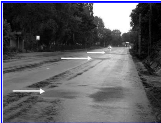
FIGURE 11.31 An example of cyclic strips of transverse porosity on a new SMA course. (Photo courtesy of Krzysztof Błażejowski.)
