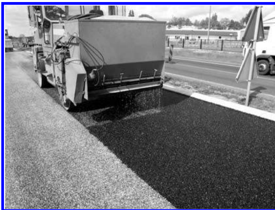
FIGURE 10.15 SMA gritters installed on rollers—the gap gritter. (Photo courtesy of Bartosz Wojczakowski.)
