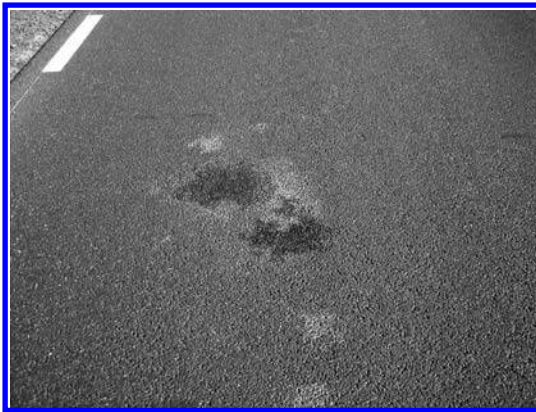
FIGURE 11.11 Seepage of water through an SMA layer. (Photo courtesy of Bohdan Dołżycki.)
