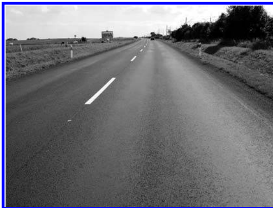
FIGURE 11.34 Mastic squeezed-out of SMA in wheel paths during trafficking of pavement. (Photo courtesy of Krzysztof Błażejowski.)
